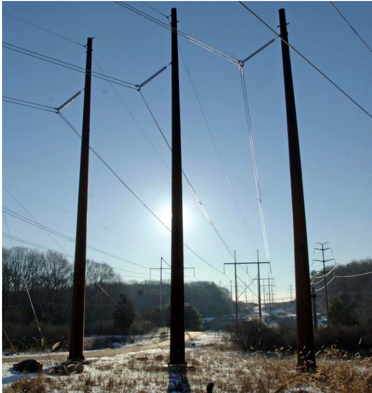
Example of weathering steel three pole (angle) structure
