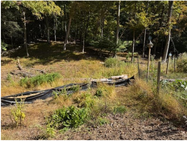
Double line of silt fence with hay bales in between. View from the west of the southern stretch. A. Moch 10/3/2025
