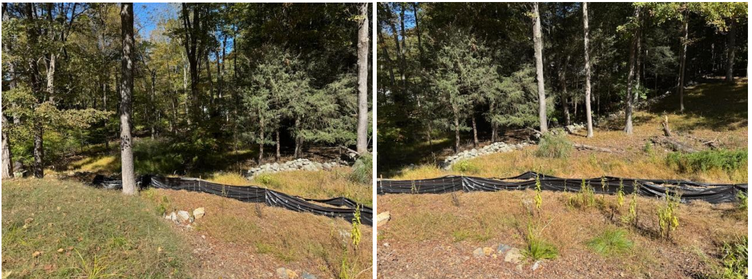
Double line of silt fence with hay bales in between. View from the west of the northern and middle section.
