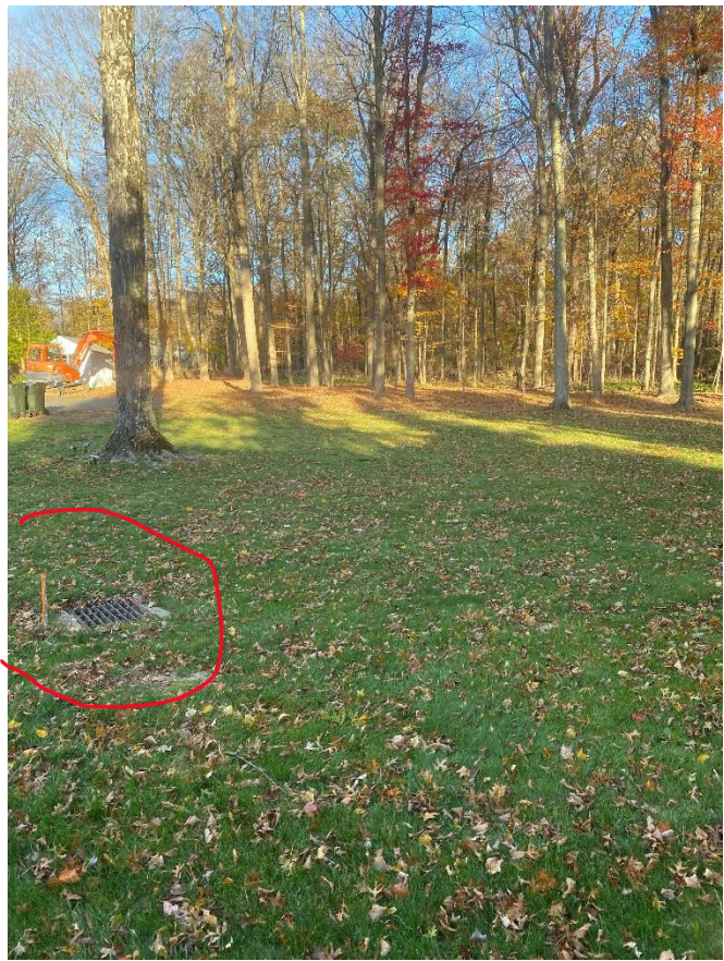
Yard drain WLF12
